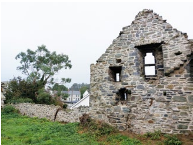
3.5.49 Missing West Section of North Elevation of Domestic Range (Insall, 2021)
