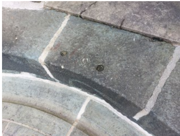
3.3.17 Showing Fixings of Missing Tracks (Insall, 2021)
