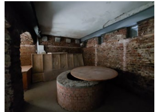
3.3.20 South Side of Ground Floor, showing well and raised ceiling level (Insall, 2021)
