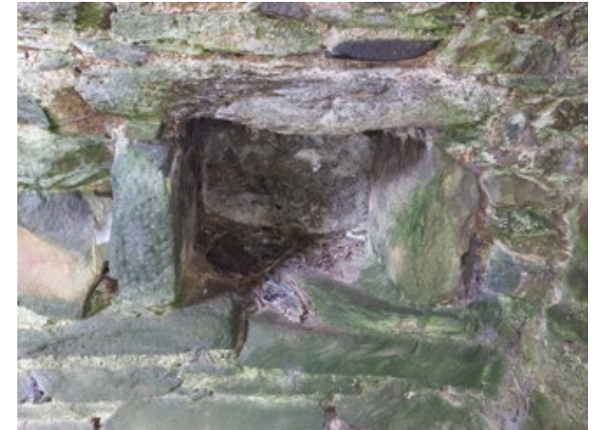
3.5.16 Wall Press, to the Rear of the Northwest Pier of the Tower (Insall, 2021)
